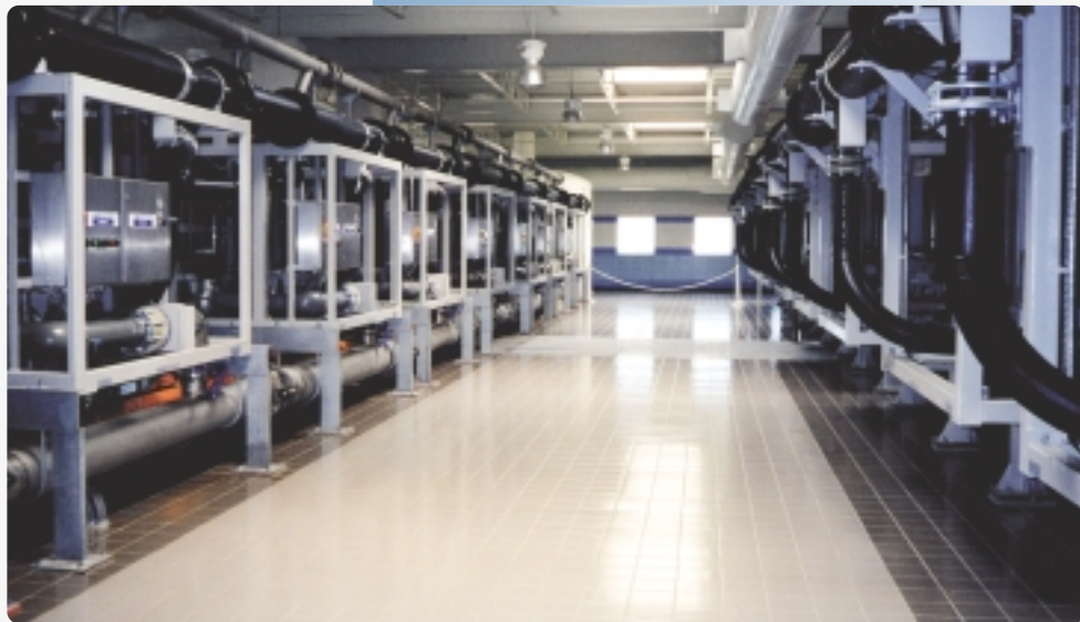
USFilter's Memcor Continuous Microfiltration (CMF) system installed at the Kenosha Water Utility treatment facility in Wisconsin.
