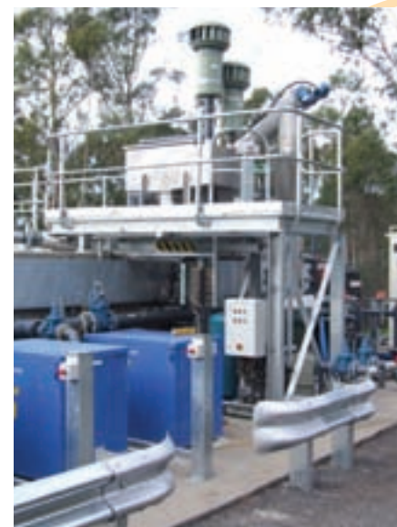
Figure 3: Cobargo MBR Plant
