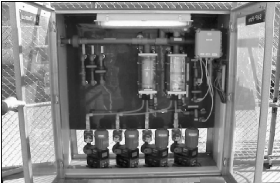
Chlorine dioxide generators can produce high levels of disinfection byproducts, but combining chlorine with chlorine dioxide can effectively disinfect water while keeping the level of disinfection byproducts low.
