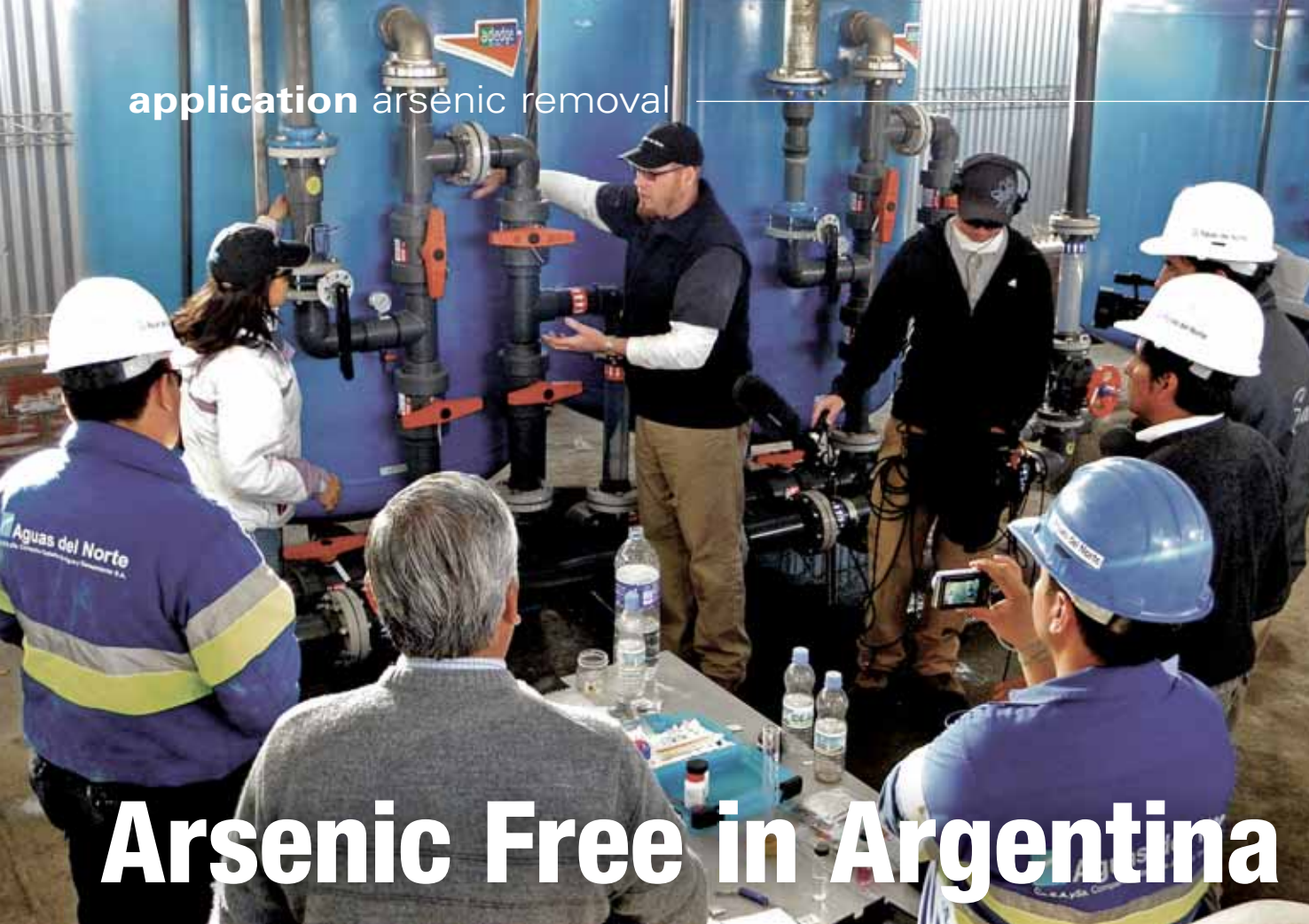
Engineers provide operator training for the new arsenic treatment system.
